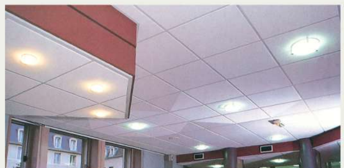
Tiles Ceiling System
