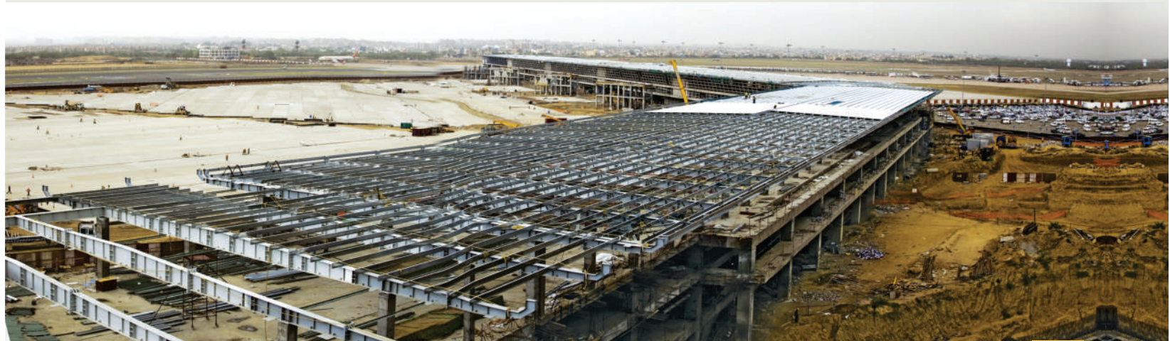
Pre-Engineered Structural Steel & Multi Layer Roofing Systems - IGI Airport Terminal 3 - Panoramic View International PIER Roof
